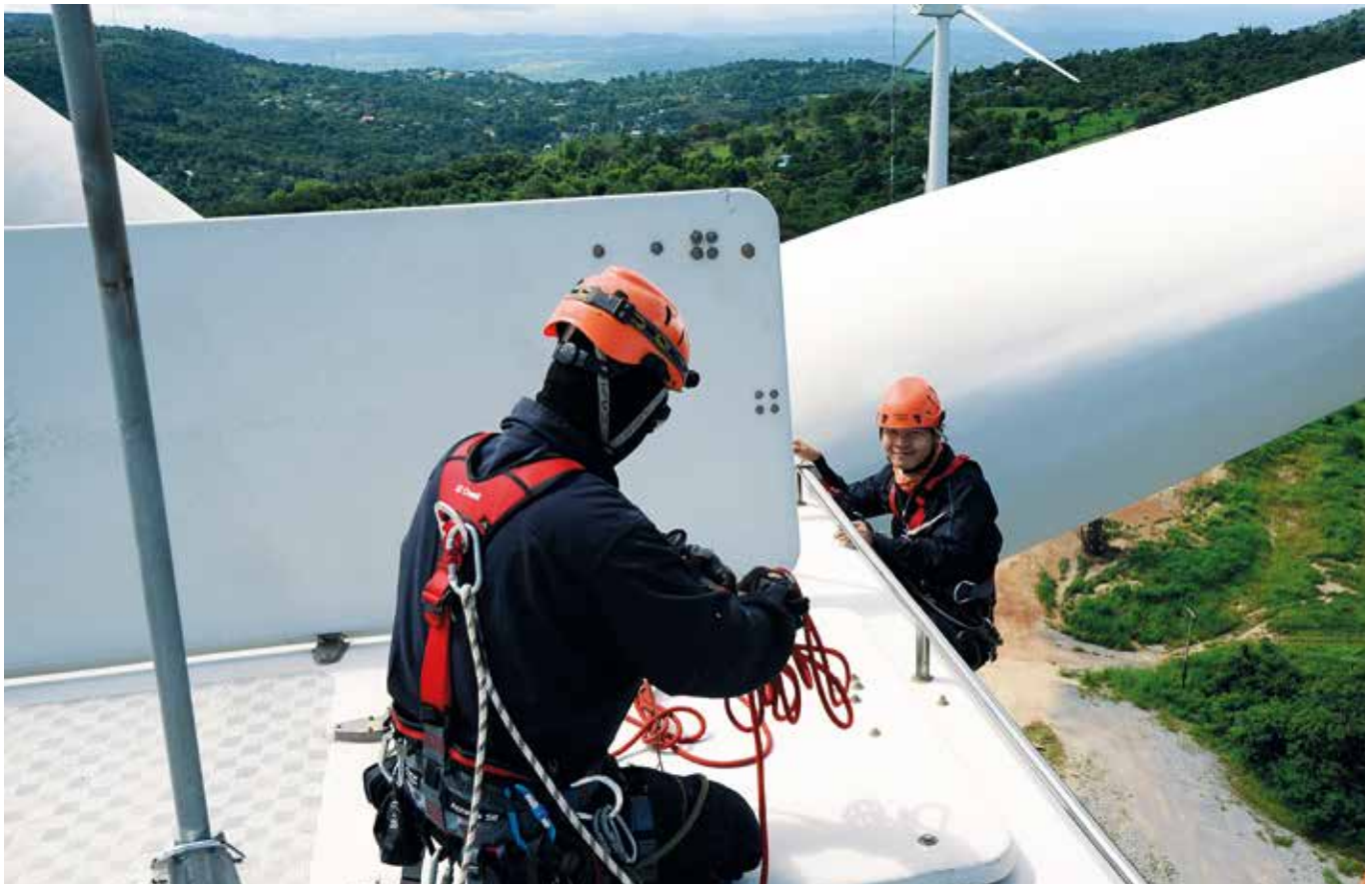
Rigging the descent from a wind turbine owned by the Electricity Generating Authority of Thailand (EGAT). Preparación para el descenso por una turbina eólica de propiedad de Electricity Generating Authority of Thailand (EGAT) Nakorn Ratchasima, Thailand (courtesy of Outdoor Solution and High Solution Network, ph. Patcharakan Babprasertth).
