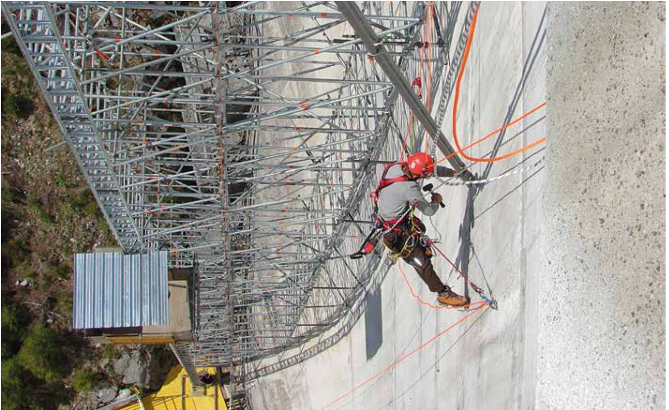
Installation of scaffolding on the Hongrin dam. Instalación de andamios para la presa de Hongrin. Vaud, Switzerland (courtesy of Corde-Access SA).
