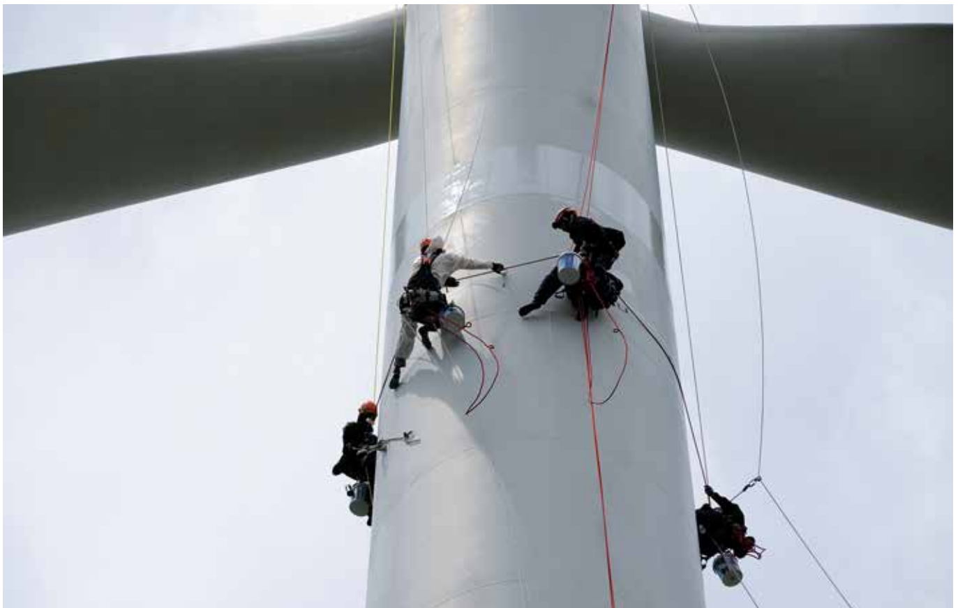
Painting a wind turbine owned by the Electricity Generating Authority of Thailand (EGAT). Operaciones de pintura de una turbina eólica de propiedad de Electricity Generating Authority of Thailand (EGAT). Nakorn Ratchasima, Thailand (courtesy of Outdoor Solution and High Solution Network, ph. Patcharakan Babprasert).
