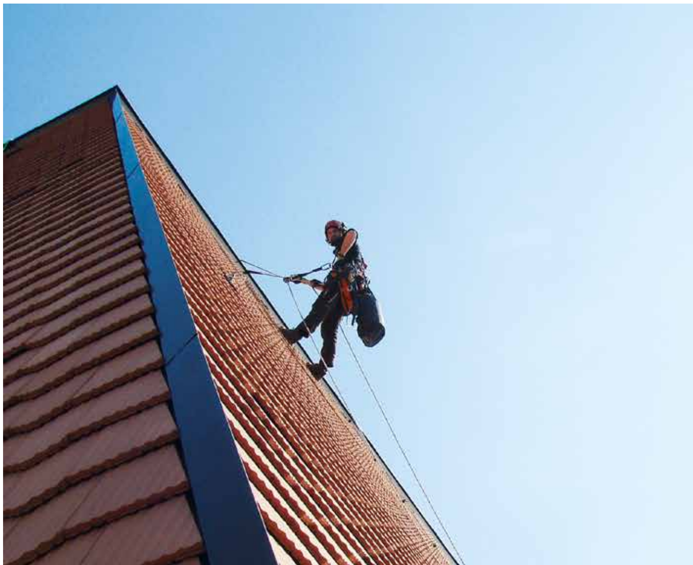
Using rope access for the control and inspection of roofing tiles. Control de las tejas de un tejado. Lausanne, Switzerland (courtesy of Corde-Access SA).
